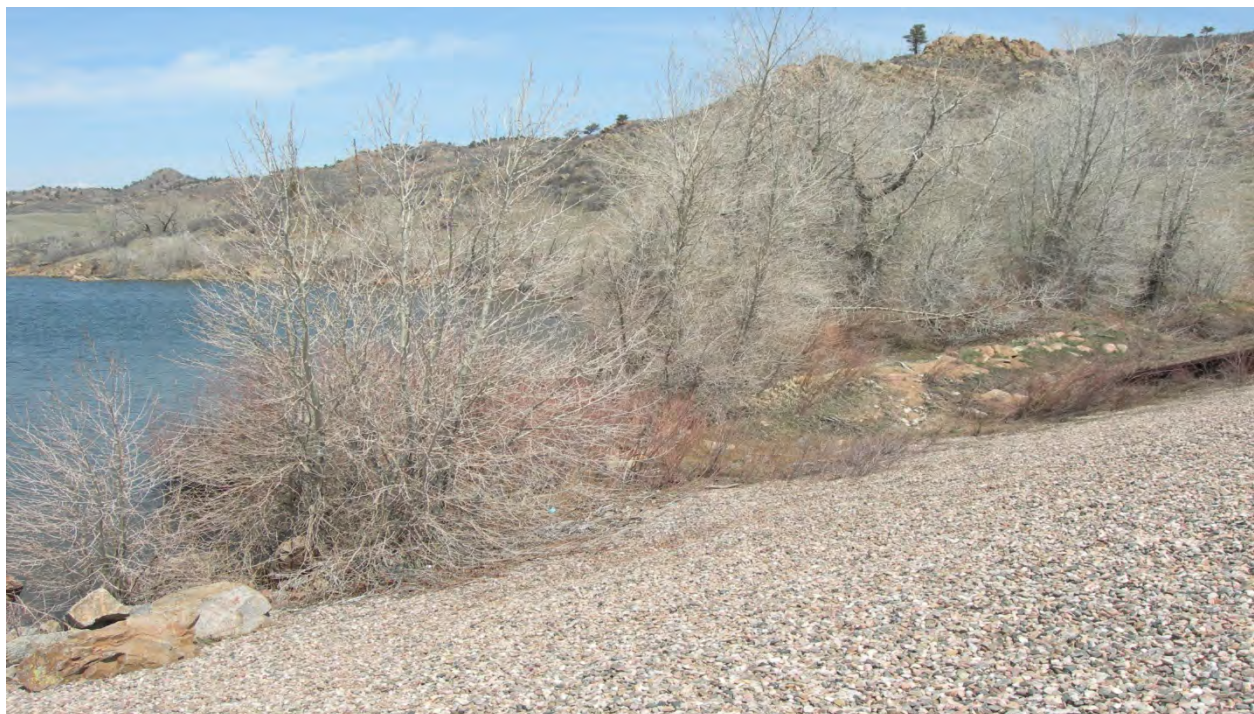
Photo 14: Trees on upstream side of northern-most fuse plug. (May 6, 2013)
