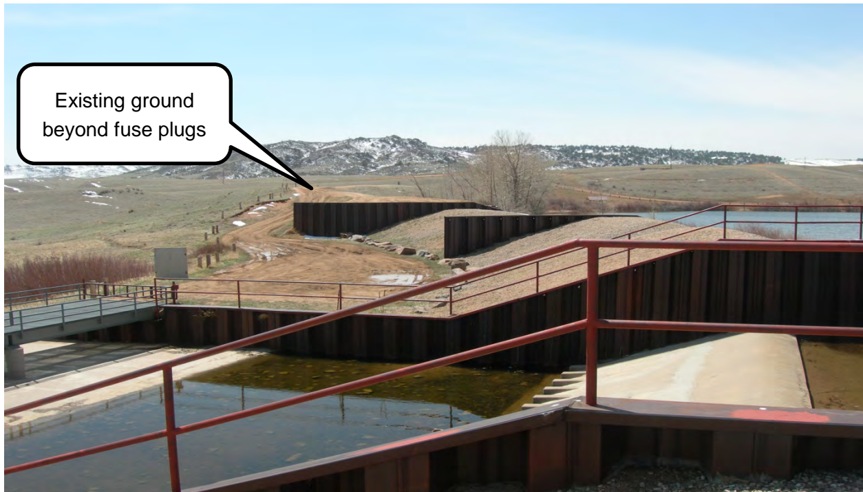
Photo 13: Looking south from northern-most fuse plug. Elevation of existing ground beyond southern-most fuse plug is only slightly above elevation of fuse plugs for several hundred yards. (May 6, 2013)
