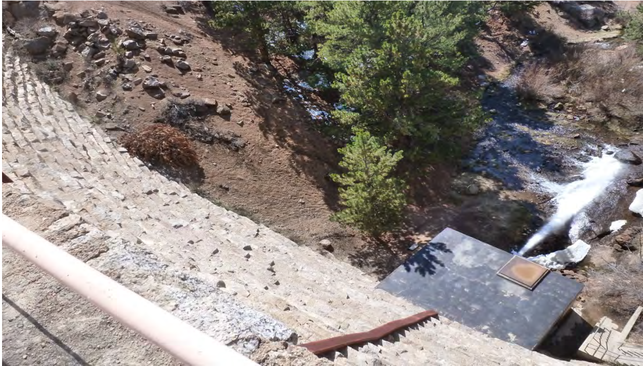
Photo 19: Left abutment of dam. Some tree and shrub growth along abutment. (May 6, 2013)
