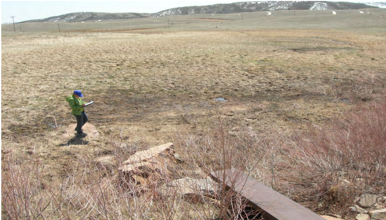
Photo 11: Large wet area downstream of spillway. Could potentially be runoff from recent snowfall. (May 6, 2013)
