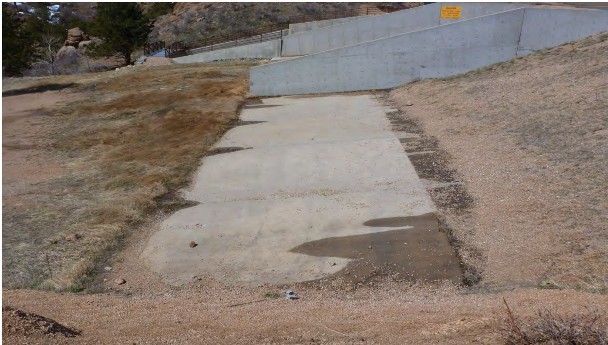
Photo 8: Downstream side of east fuse plug. Minor seepage coming from underneath fuse plug material and through concrete base construction joints. (May 6, 2013)
