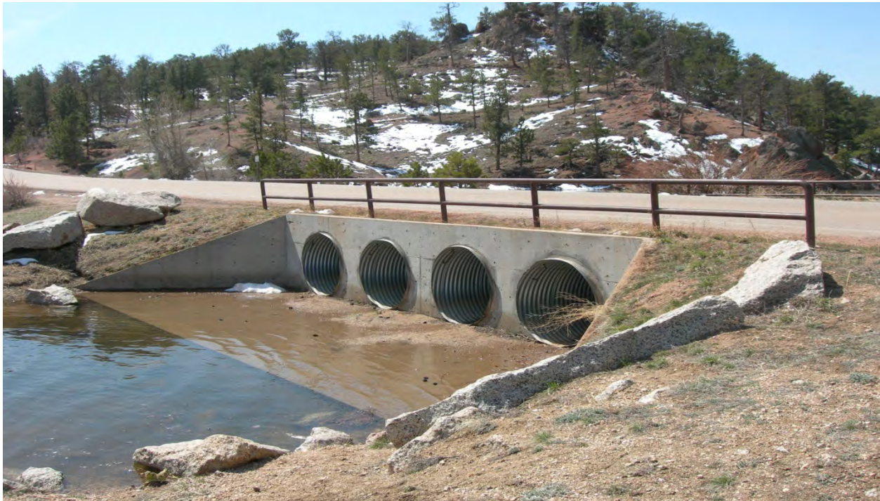
Photo 39: Culverts running under a land bridge near where Middle Crow Creek meets Granite Springs Reservoir. (May 6, 2013)
