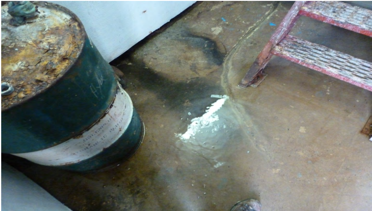
Photo 34: Standing water on floor of outlet works building. (May 6, 2013)
