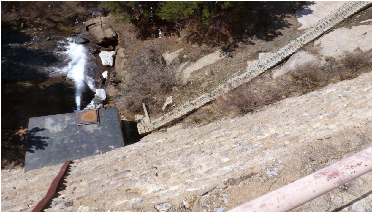
Photo 21: Right abutment of dam. Outlet works building. Some shrub growth along the abutment. (May 6, 2013)
