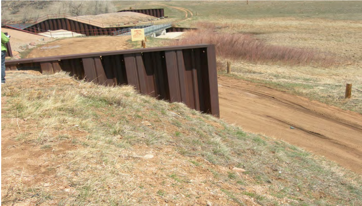
Photo 5: Downstream slope of right abutment of southern-most fuse plug. Slope approximately 1H:1V or steeper. (May 6, 2013)
