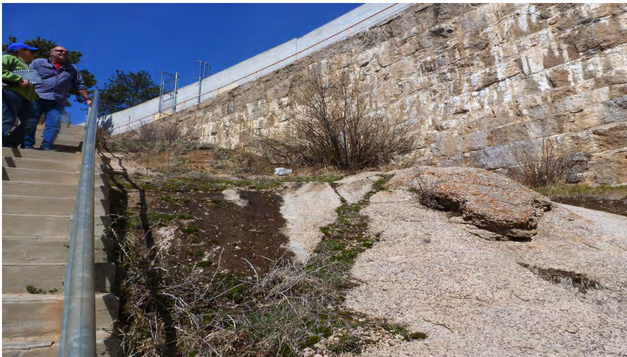
Photo 22: Minor seepage along right abutment. Starts at wall interface. (May 6, 2013)
