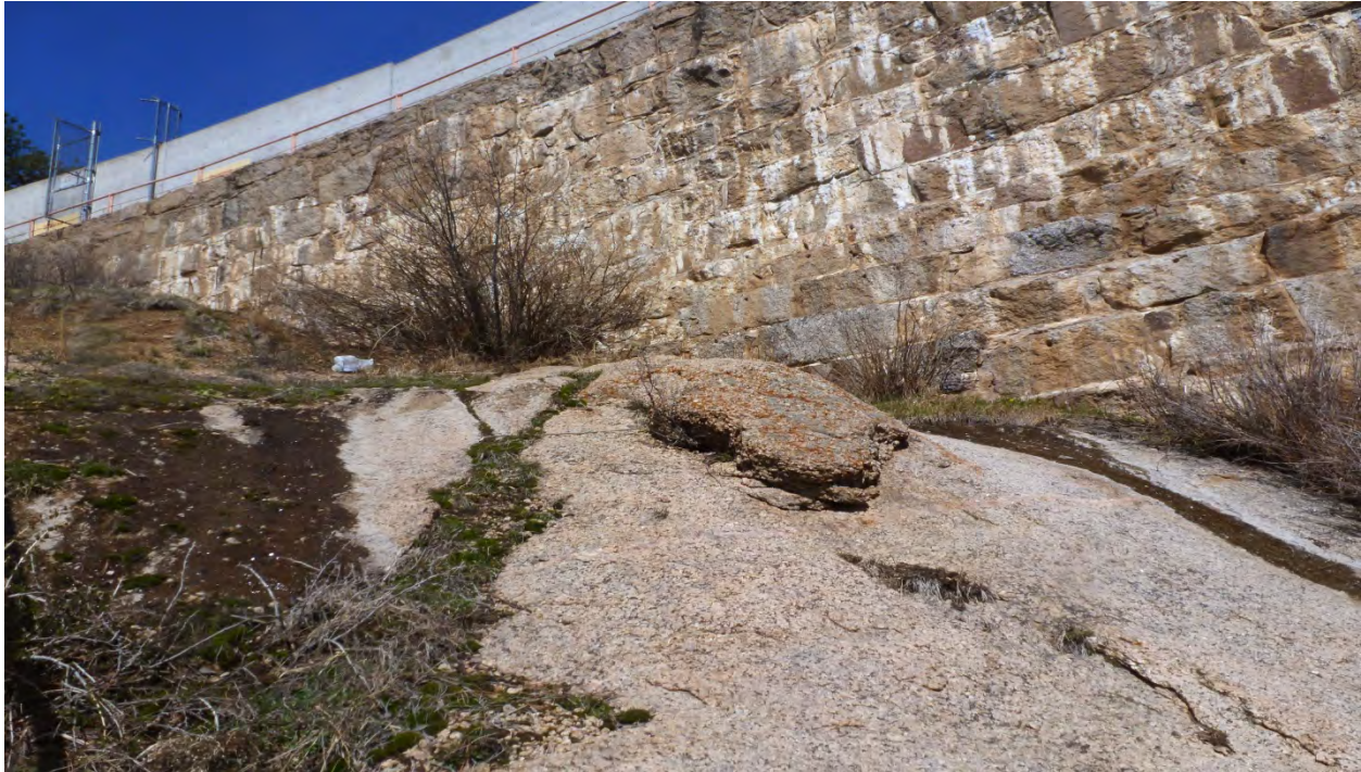
Photo 23: Minor seepage along right abutment. Starts at wall interface. (May 6, 2013)
