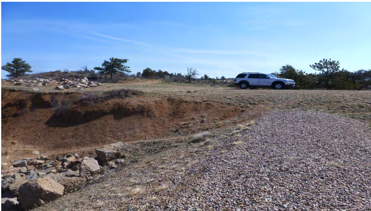
Photo 2: From left-most fuse plug, looking northeast at fuse plug left abutment (spillway release guide dike). (May 6, 2013)
