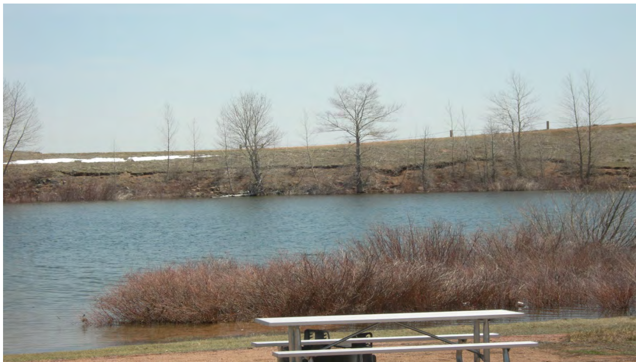
Photo 2: Sloughing of existing ground to the right of the fuse plugs. (May 6, 2013)
