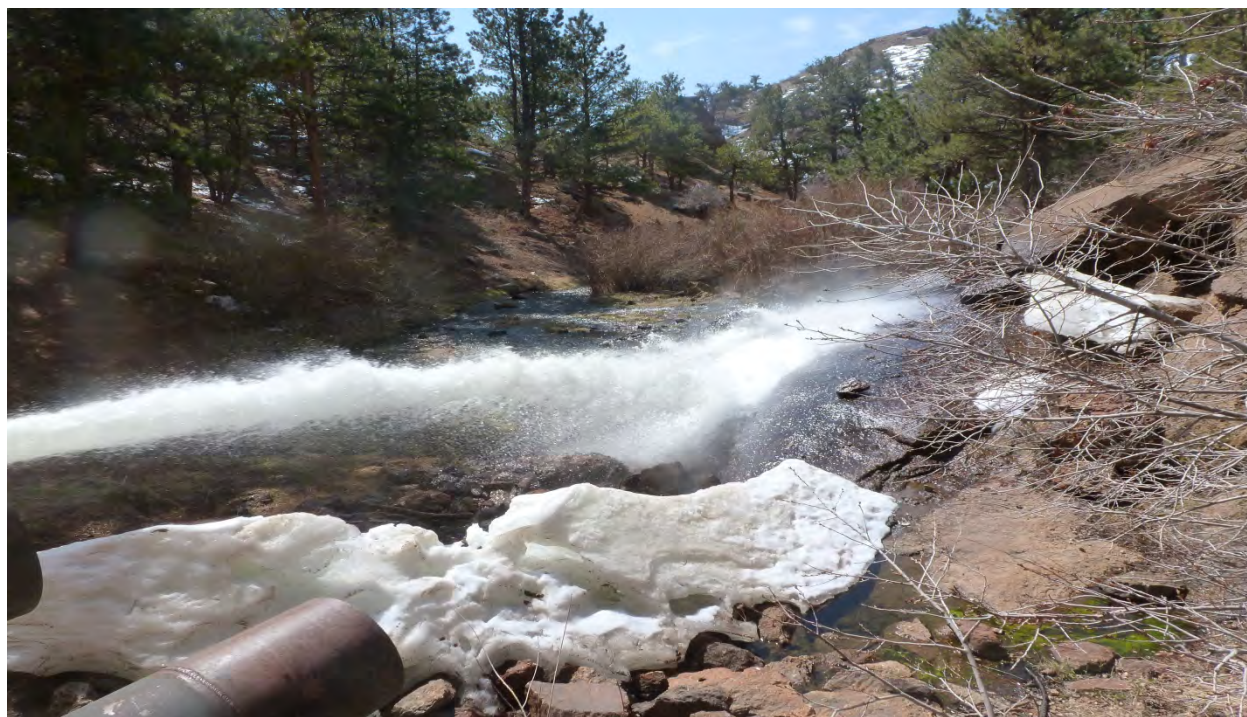
Photo 32: Downstream of outlet works. Water falls directly onto exposed granite. (May 6, 2013)
