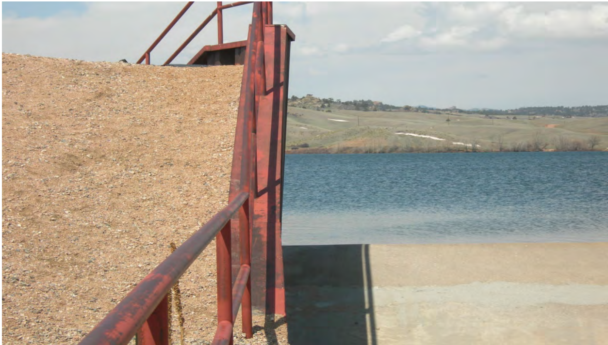
Photo 8: Right abutment wall of spillway is bulging slightly inward. (May 6, 2013)
