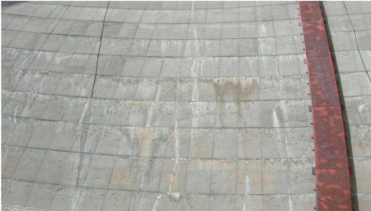
Photo 29: Downstream face of dam right of centerline. Some calcium deposits forming at joints. (May 6, 2013)
