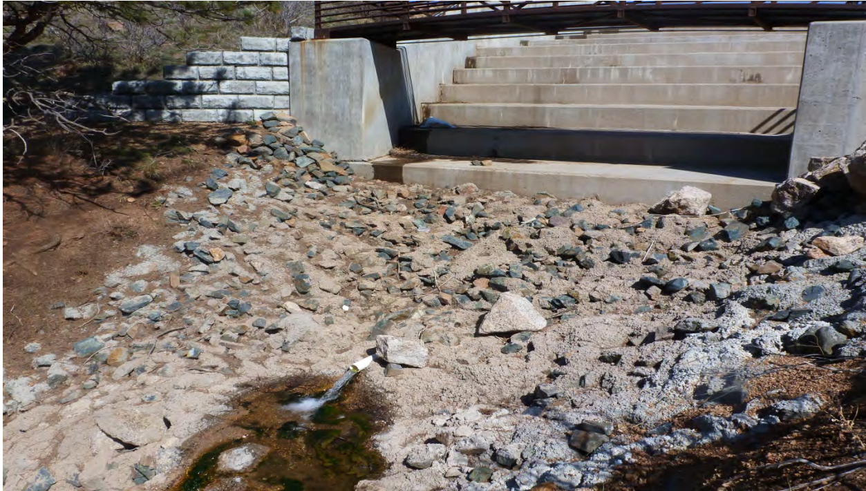
Photo 11: Downstream of main spillway. Notice spillway subdrain system outfall pipe, flowing approximately 20 gpm. Riprap is grouted in. (May 6, 2013)
