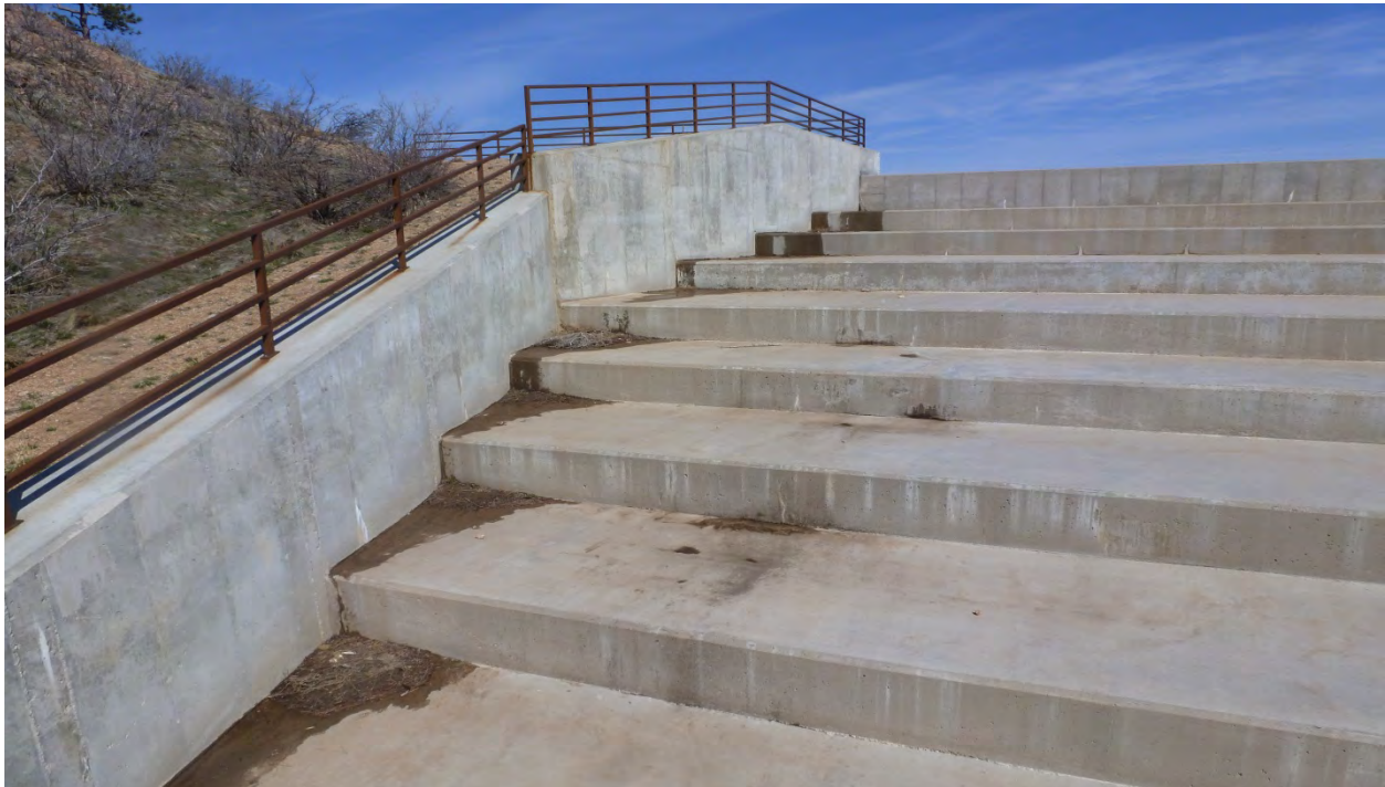
Photo 10: Granite Springs main spillway looking upstream. Minor seepage along west wall. (May 6, 2013)
