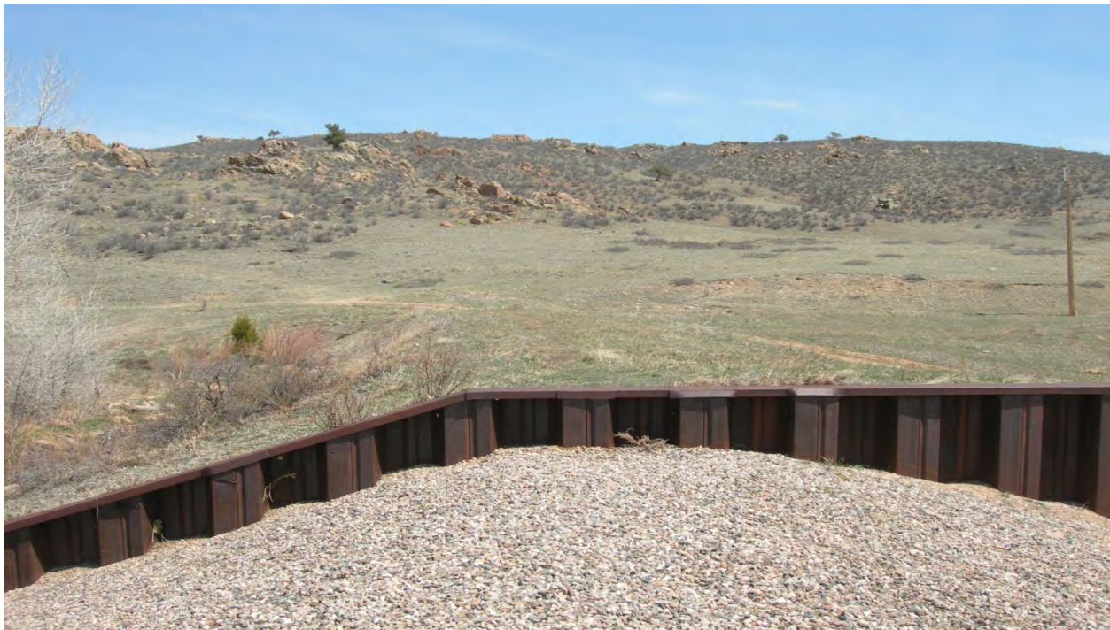
Photo 12: Embankment to the north of the northern-most fuse plug. Slightly above the elevation of the fuse plugs for 100-200 yards. (May 6, 2013)
