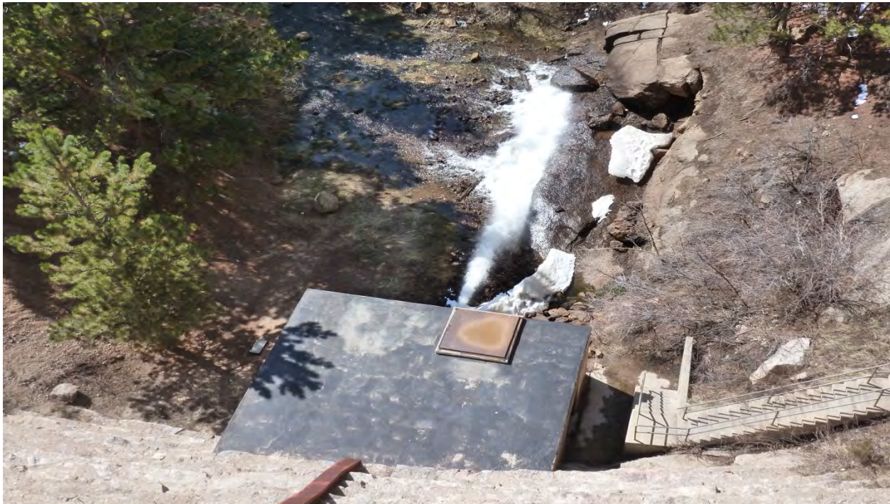
Photo 24: Downstream toe of dam. Outlet works building. Some trees and shrubs. (May 6, 2013)
