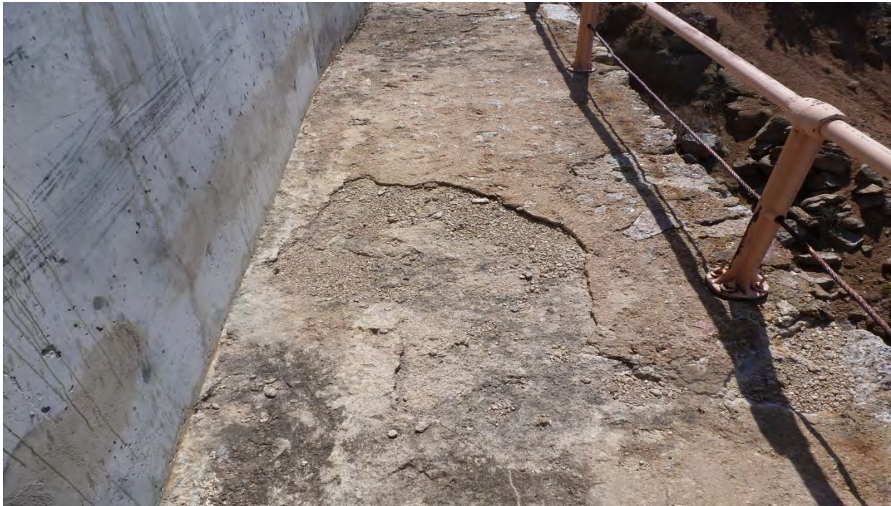
Photo 16: Dam crest, typical. Some deterioration. (May 6, 2013)
