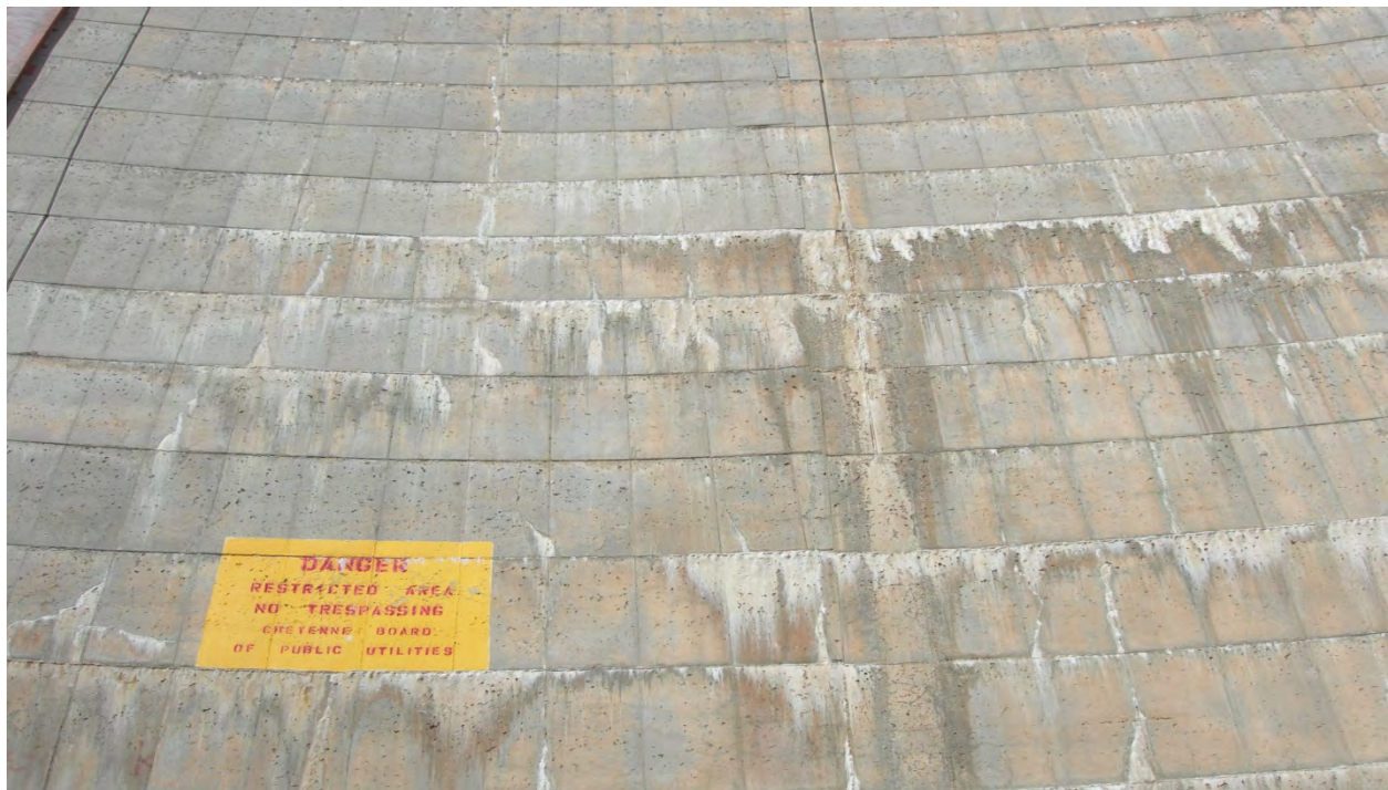
Photo 28: Downstream face of dam left of centerline. Some calcium deposits forming at joints. (May 6, 2013)
