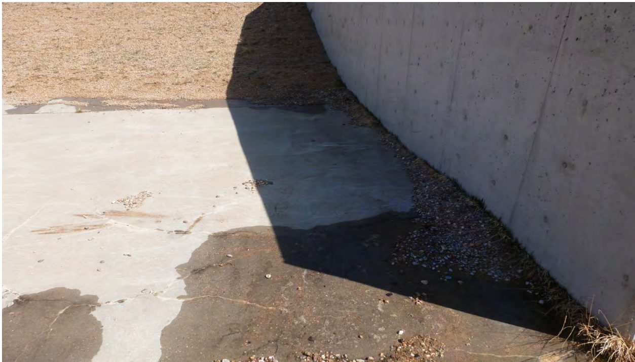
Photo 6: Downstream side of west fuse plug. Seepage coming from underneath fuse plug material. (May 6, 2013)
