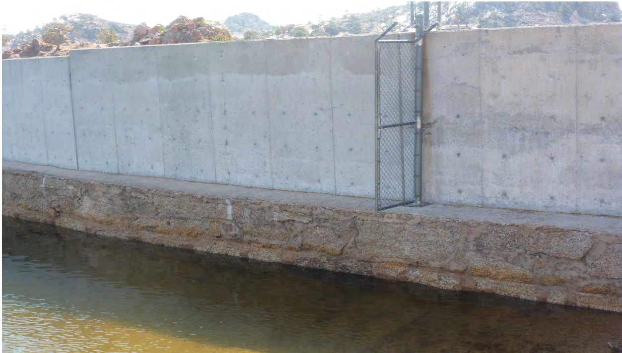
Photo 26: Upstream face of dam, typical. Notice high water mark approximately 1 foot above current pool elevation. (May 6, 2013)
