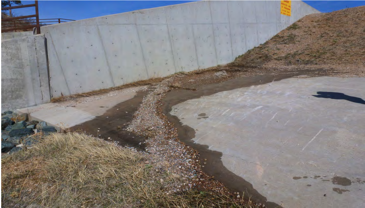
Photo 5: Downstream side of west fuse plug. Seepage coming from underneath fuse plug material. (May 6, 2013)
