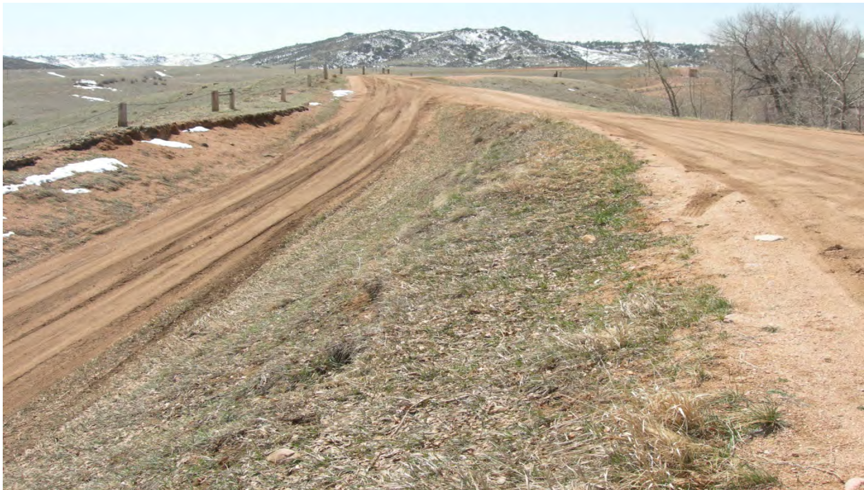
Photo 4: Downstream slope of right abutment of southern-most fuse plug. Slope approximately 1H:1V or steeper.
