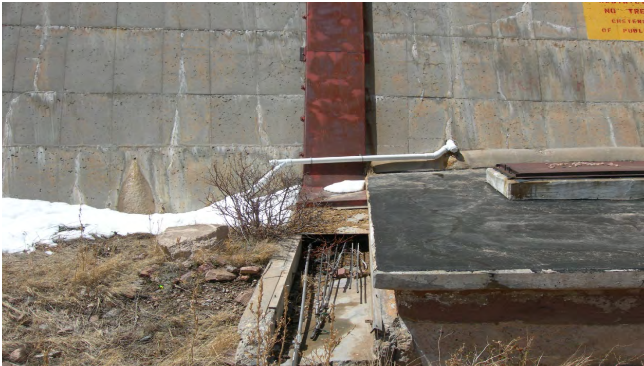
Photo 24: Roof of outlet works building. Internal seepage pipe was rerouted (as shown) because it was regularly releasing water onto the roof. (May 6, 2013)
