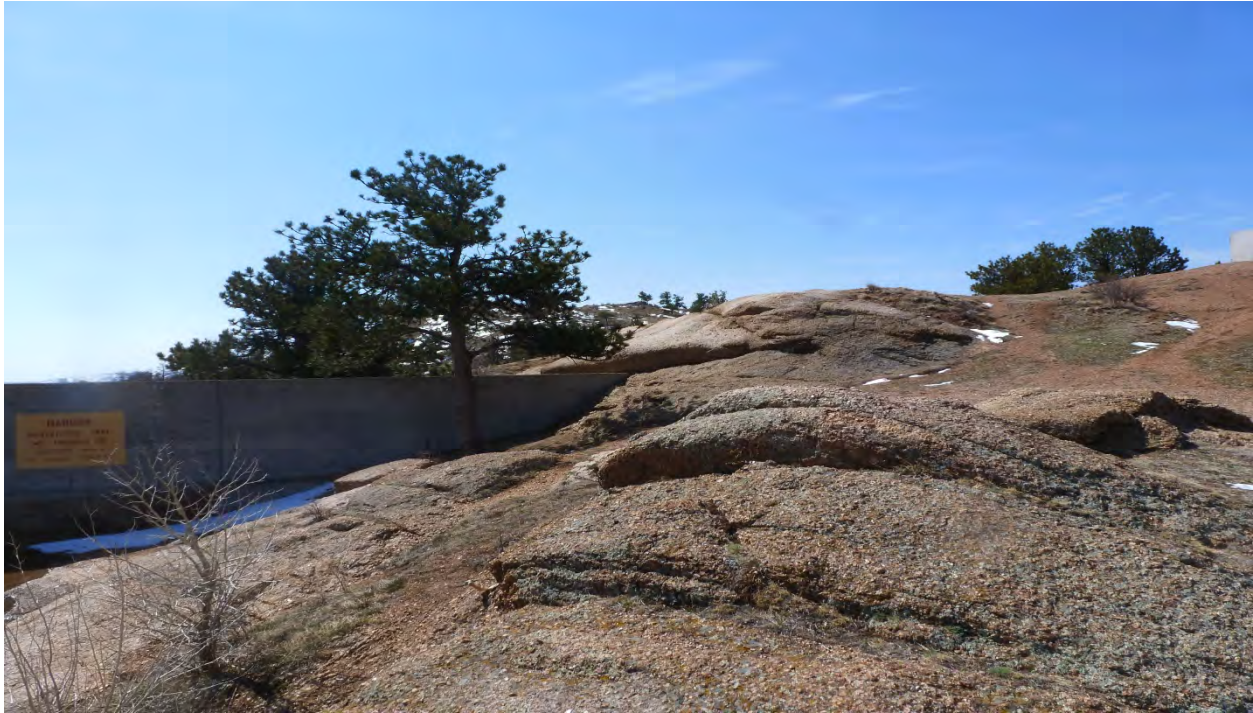
Photo 29: Upstream of right abutment of dam looking downstream to the south. (May 6, 2013)
