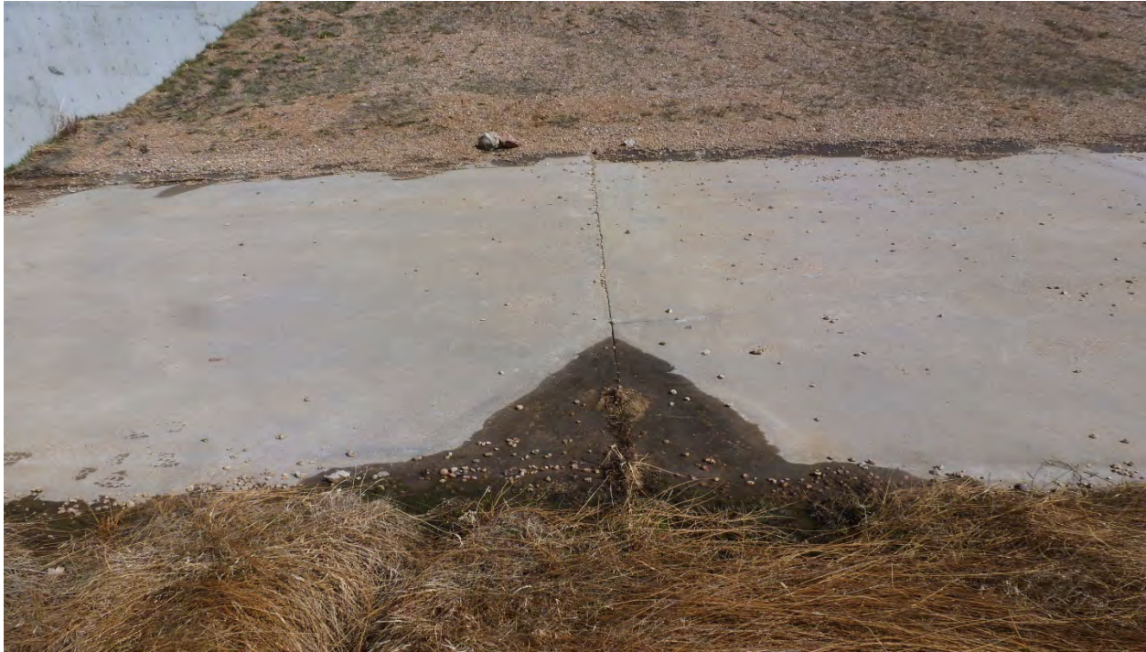
Photo 7: Downstream side of east fuse plug. Minor seepage coming through concrete base construction joints.
