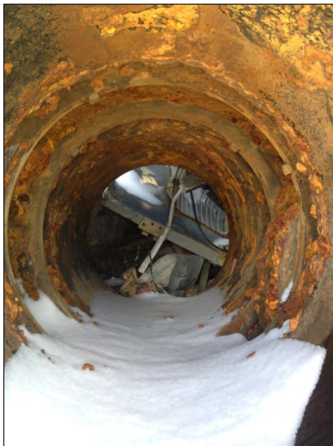
Figure Error! No text of specified style in document..2 Evidence of tuberculation inside scraped water main
